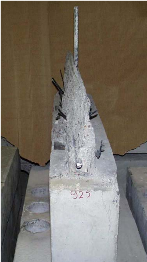
Fig. 19. Uncracked joint concrete on top of the upper wall element seen from south.
