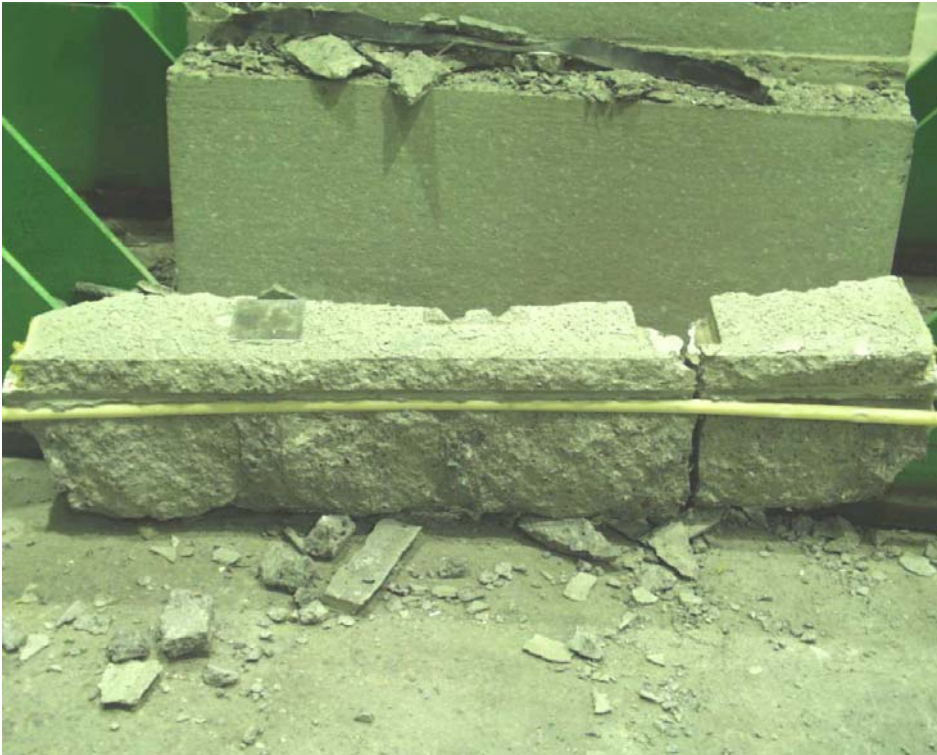
Fig. 21. A monolithic block (joint concrete) which was broken when falling down from the top of the lower wall element, seen from east.
