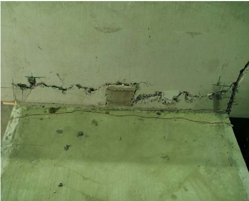
Fig. 12. Cracking pattern in the upper wall element after failure seen from west.
