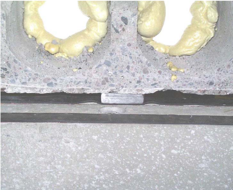
Fig. 1. Steel plate between neoprene strip and slab. Note the curvature of the strip close to the plate.
