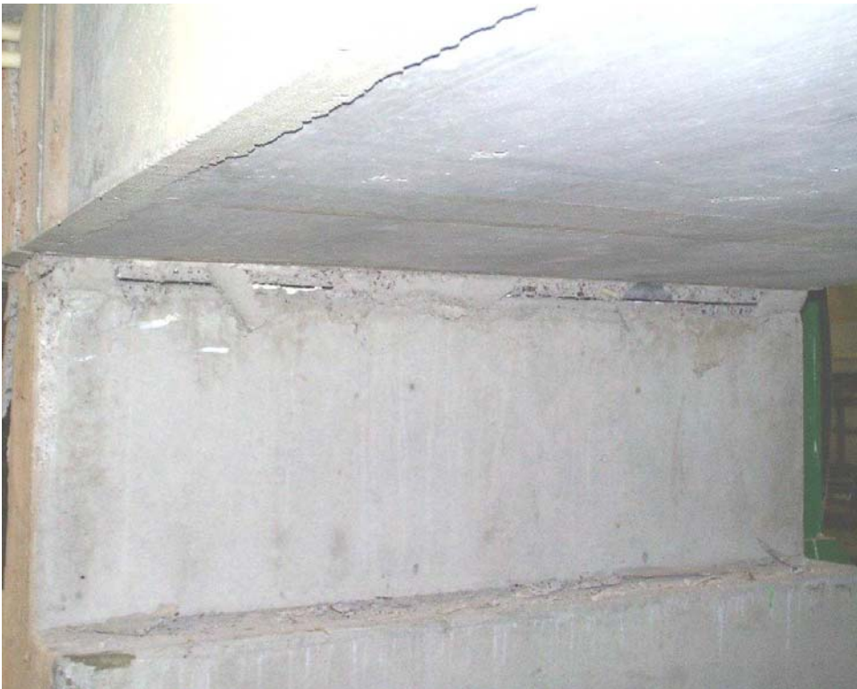
Fig. 8. Peeling of concrete in lower wall element seen from west.
