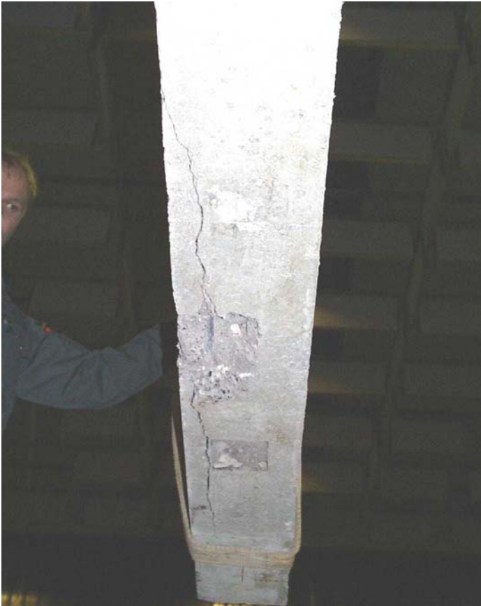
Fig. 11. Cracking pattern in upper wall element. Western face on the left.
