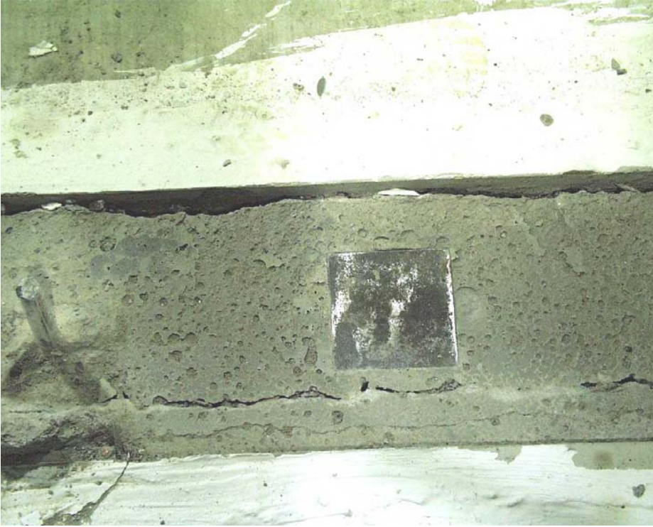
Fig. 17. Top surface of the joint after removal of the upper wall element. Note the air pores.
