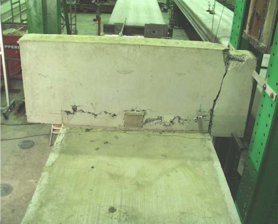
Fig. 13. Cracking pattern in the upper wall element after failure seen from west. Note also the failure of the cantilevered end which took place after step 44.
