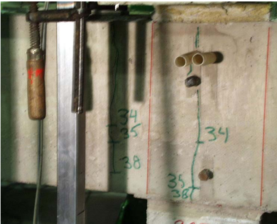
Fig. 8. Cracks at step 38 seen from north.
