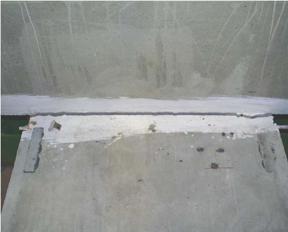
Fig.15. Uncracked eastern face of the upper wall element after failure.
