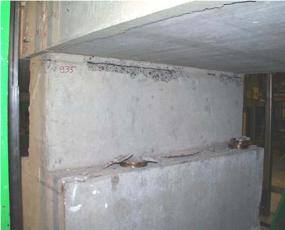
Fig. 7. Peeling of the concrete below and above the neoprene strip before failure seen from west.
