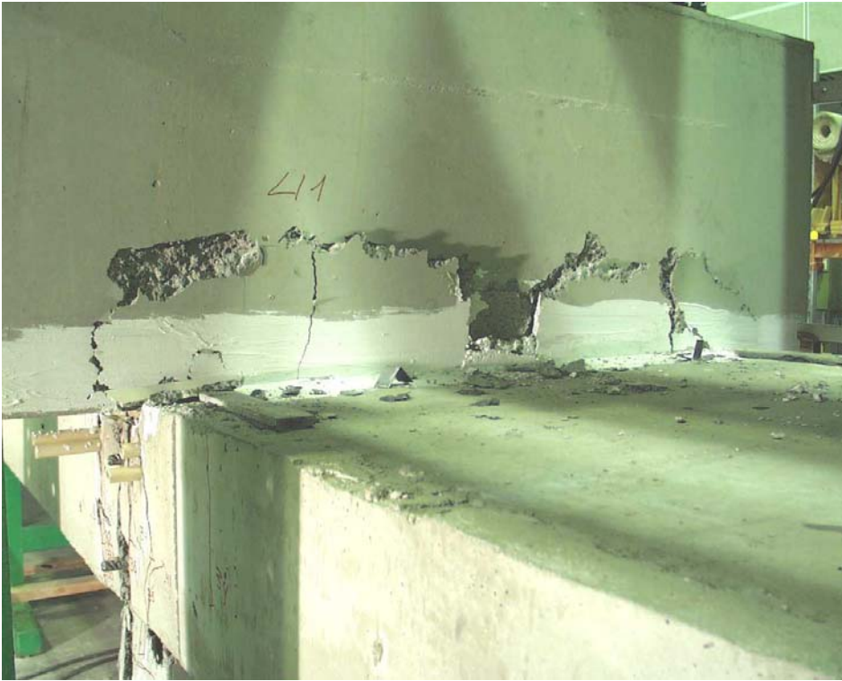
Fig. 11. Upper wall element after failure seen from west.
