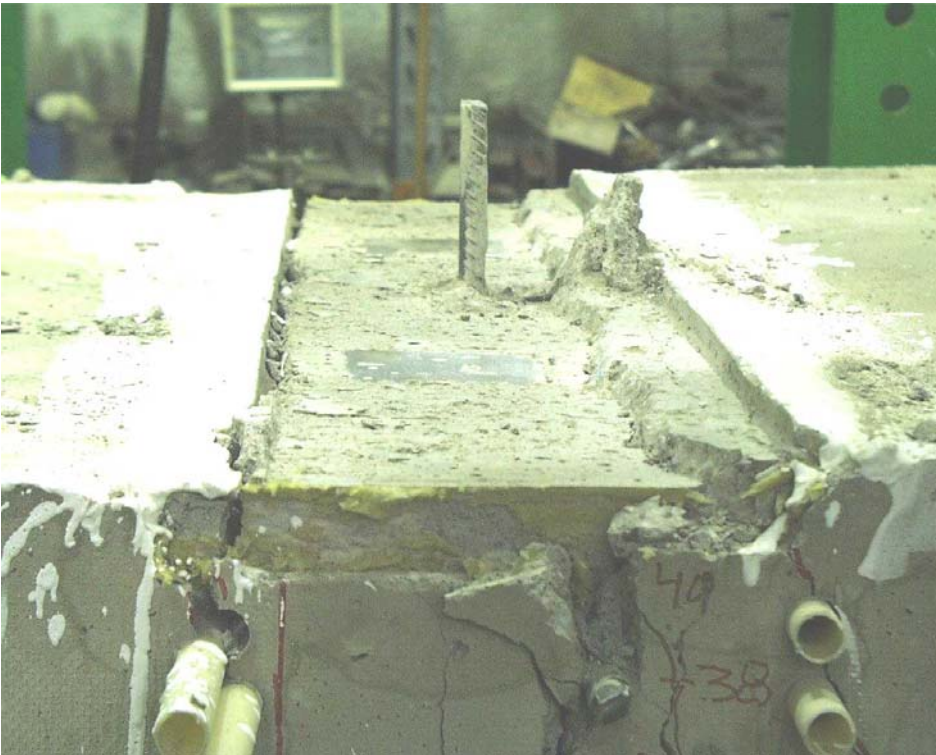
Fig. 18. Top surface of the joint after removal of the upper wall element seen from north.
