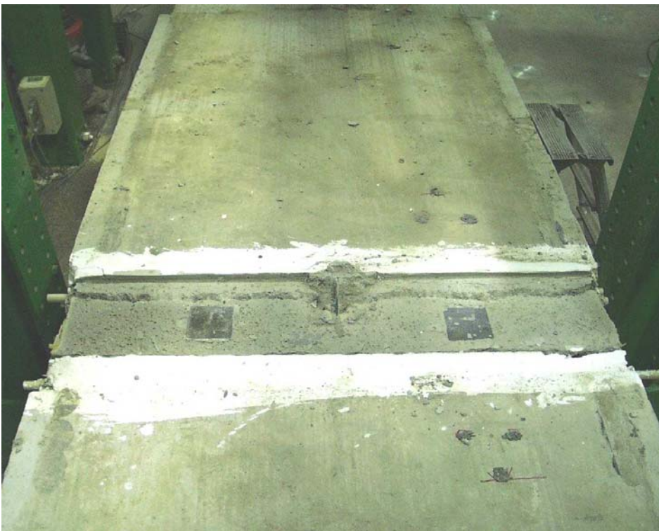
Fig. 16. Top surface of the joint after removal of the upper wall element.
