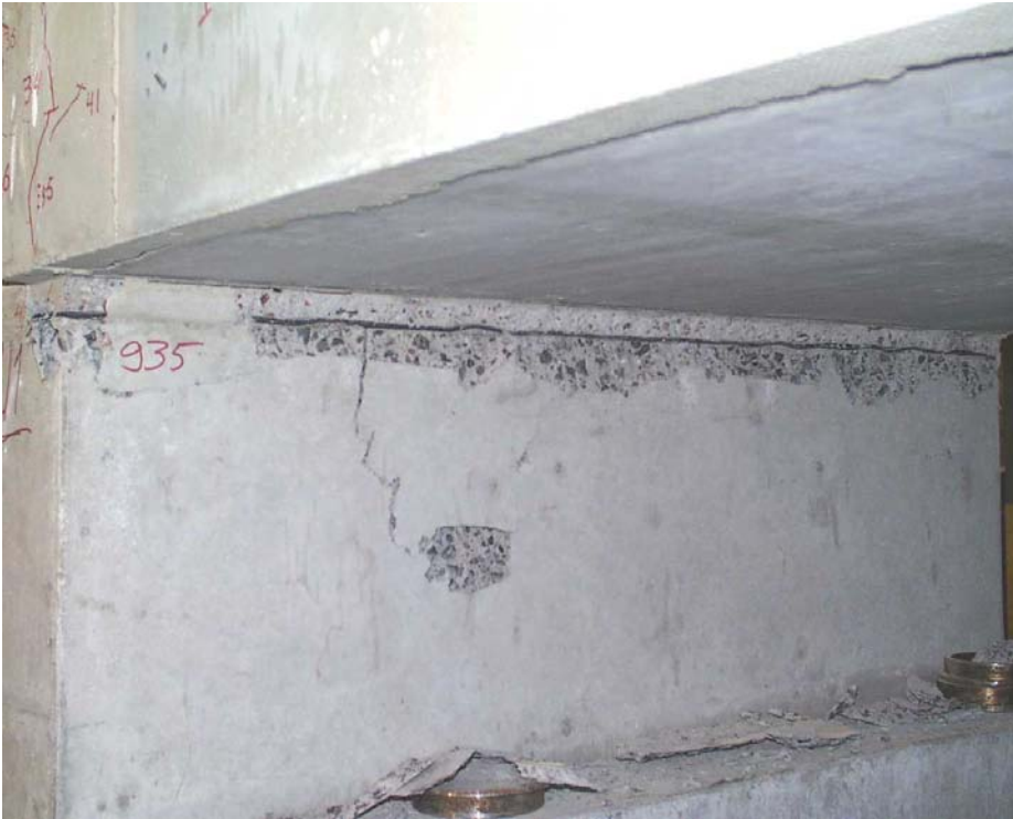
Fig. 13. Lower wall element after failure seen from west.
