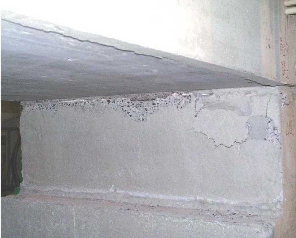
Fig. 7. Peeling of concrete in lower wall element seen from east.
