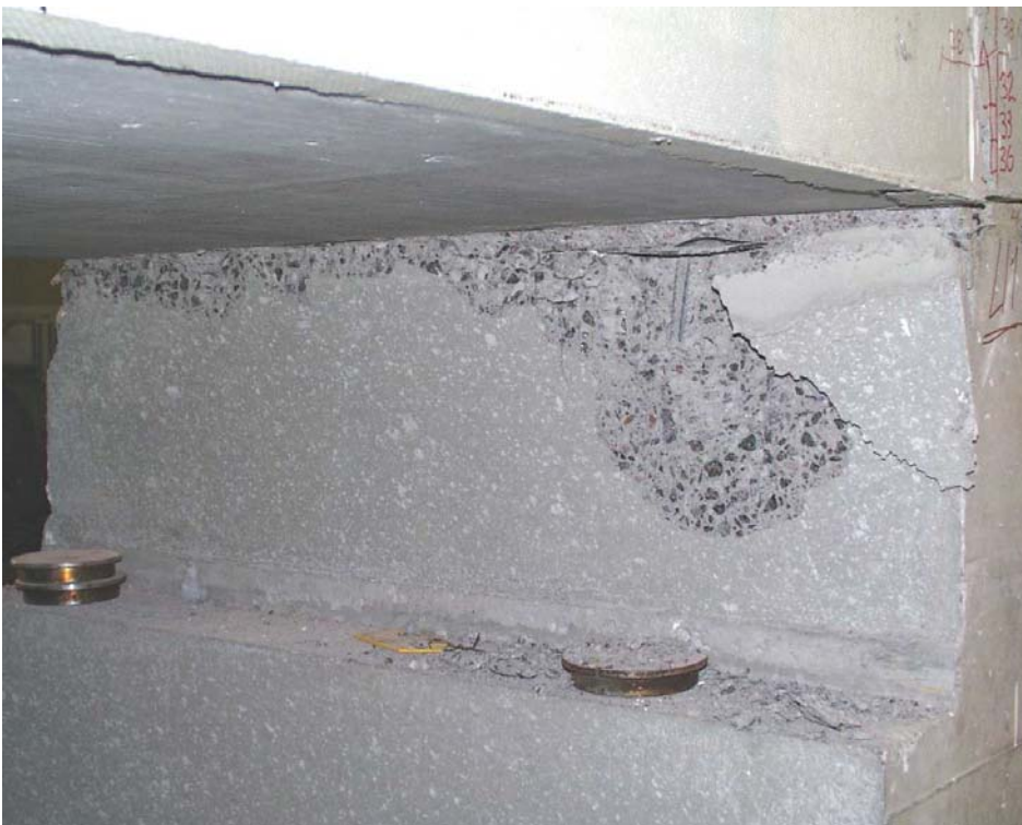
Fig. 14. Lower wall element after failure seen from east.
