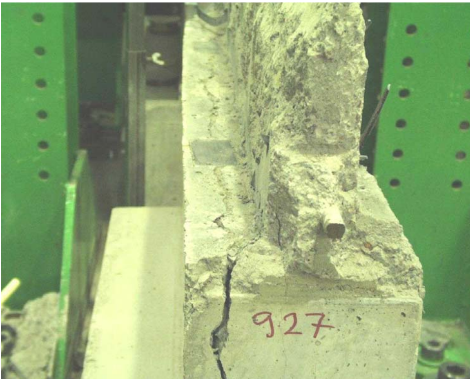
Fig. 18. Uncracked joint concrete on top of the upper wall element seen from north.
