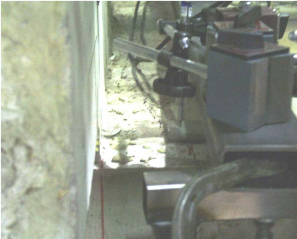
Fig. 9. Transverse crack on the top of the western slab at step 38.
