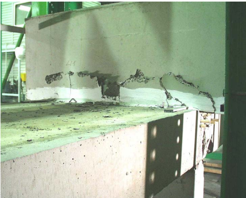
Fig. 12. Upper wall element after failure seen from west.
