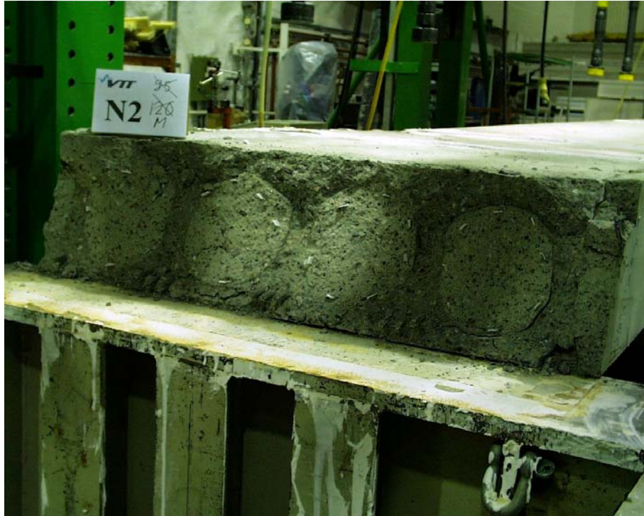
Fig. 33. N2. Flexural crack.
