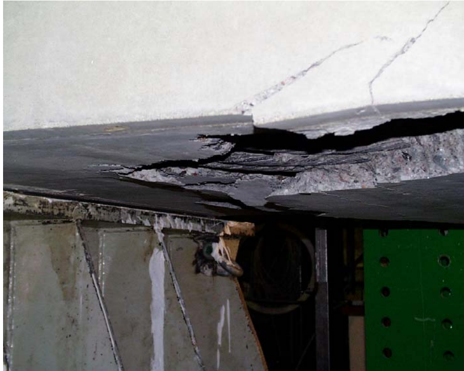
Fig. 31. N2. Soffit after failure.
