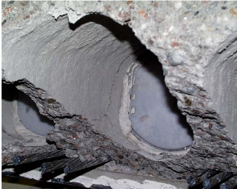
Fig. 47. B3. Detail of shear crack.
