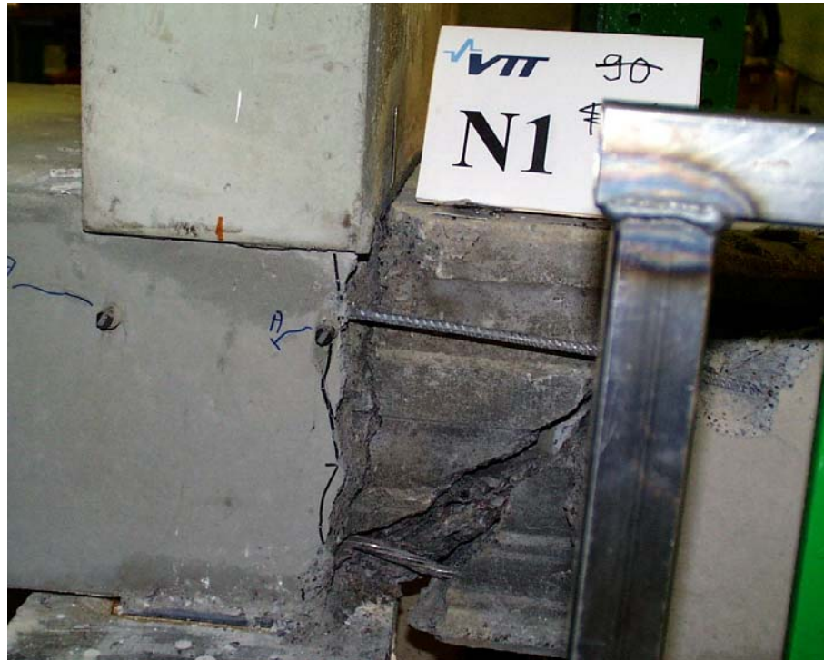
Fig. 19. N1. North edge after failure and removal of a loose piece of cast-in-situ concrete.
