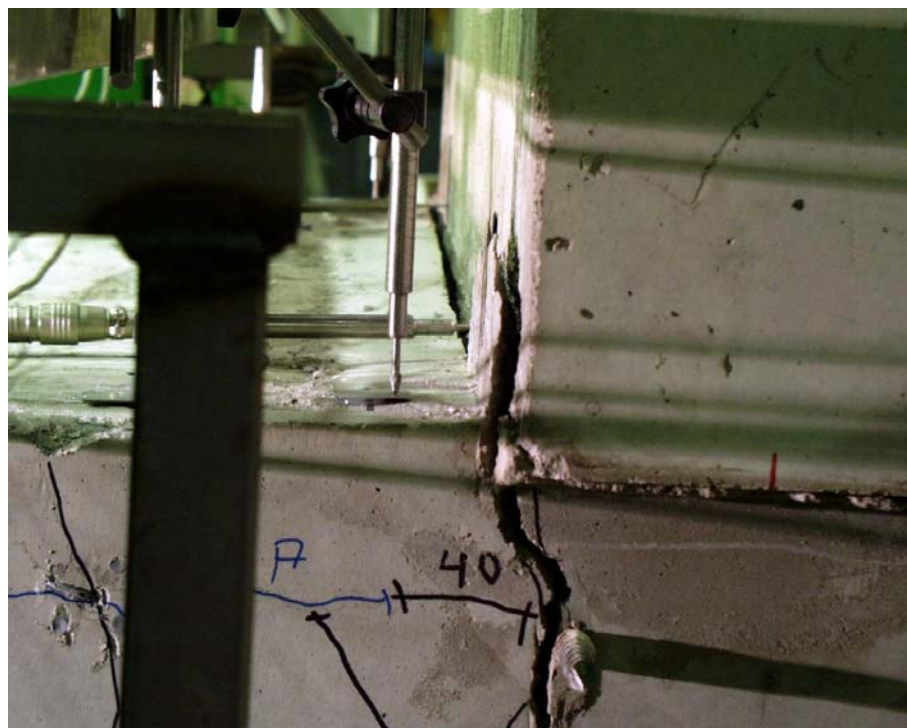
Fig. 12. N1, South edge. Flexural crack before failure.
