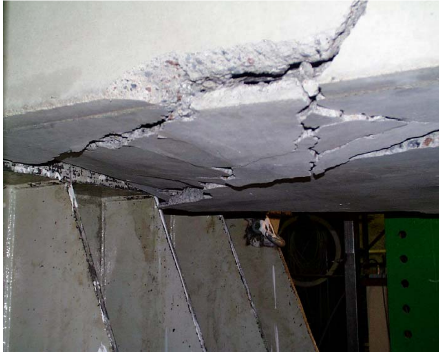
Fig. 17. N1. Soffit after failure.
