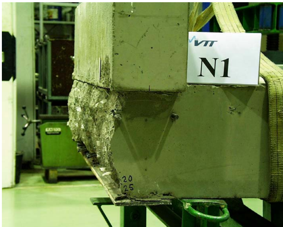
Fig. 22. N1. Vertical crack.
