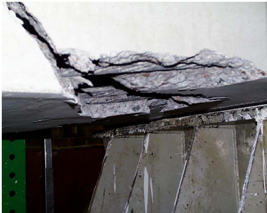
Fig. 32. N2. Soffit after failure.
